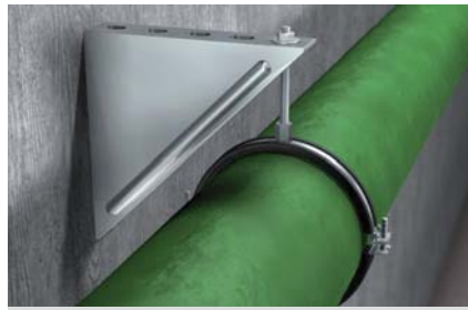
Suspended pipe under angle bracket
