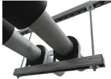
Suspended pipe support
