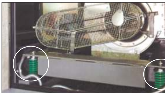
Blower in AHU on Open Spring Units
